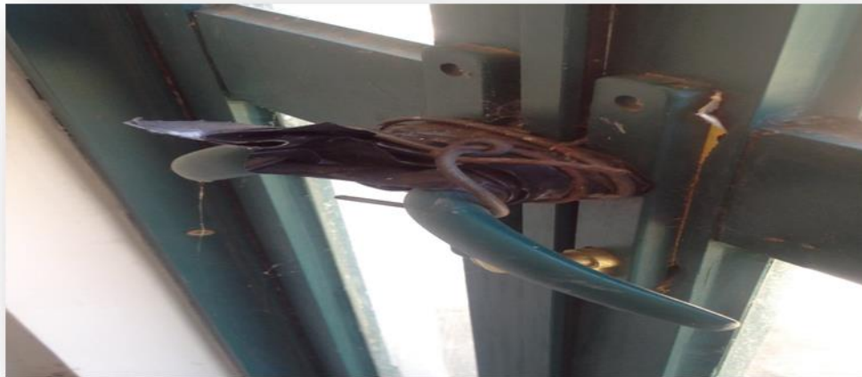
Figure 3: Exit door locked with wire in the hostel.
